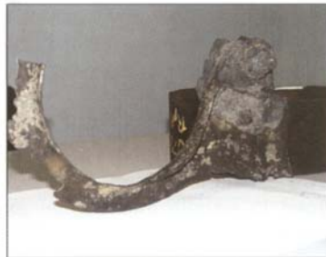
Corroded roof hanger.
