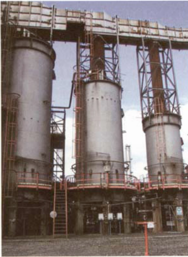
Figure 4a Vertical cylindrical furnaces.
