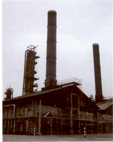
Figure 5a Multiple box type furnaces.
