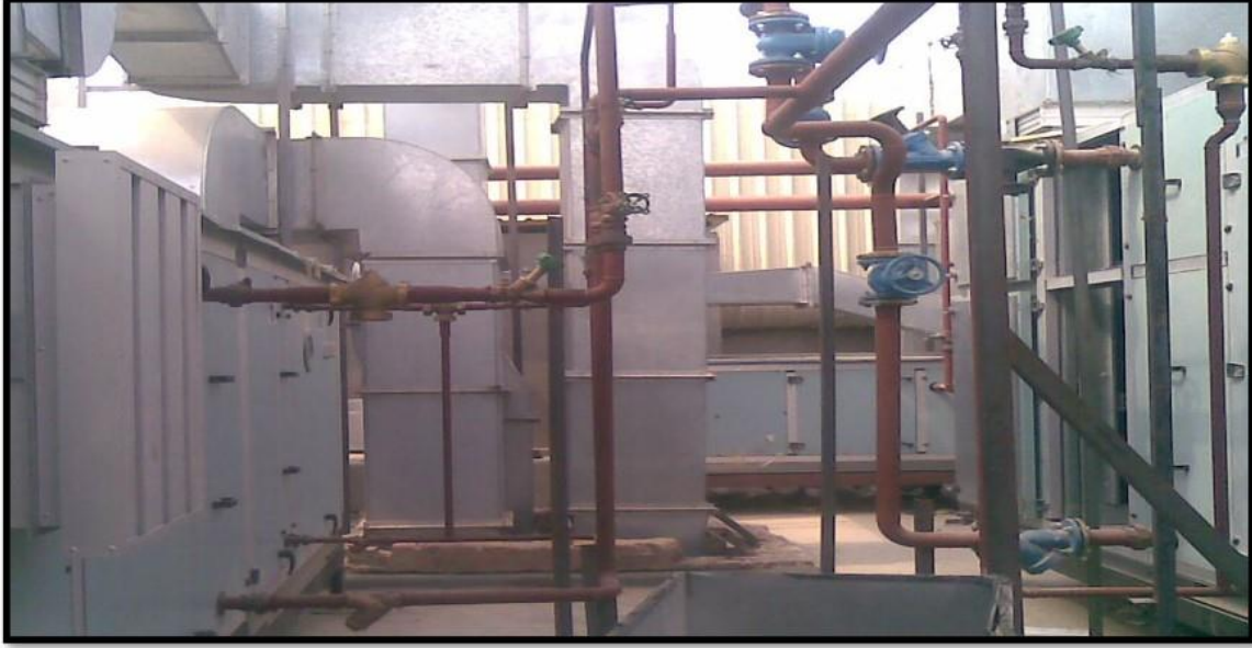
AHU outside building (at roof)
