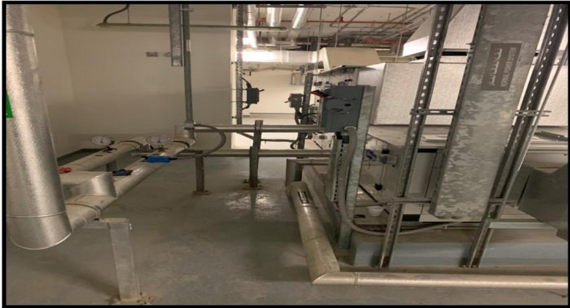
AHU Inside Building (Mechanical Room)
