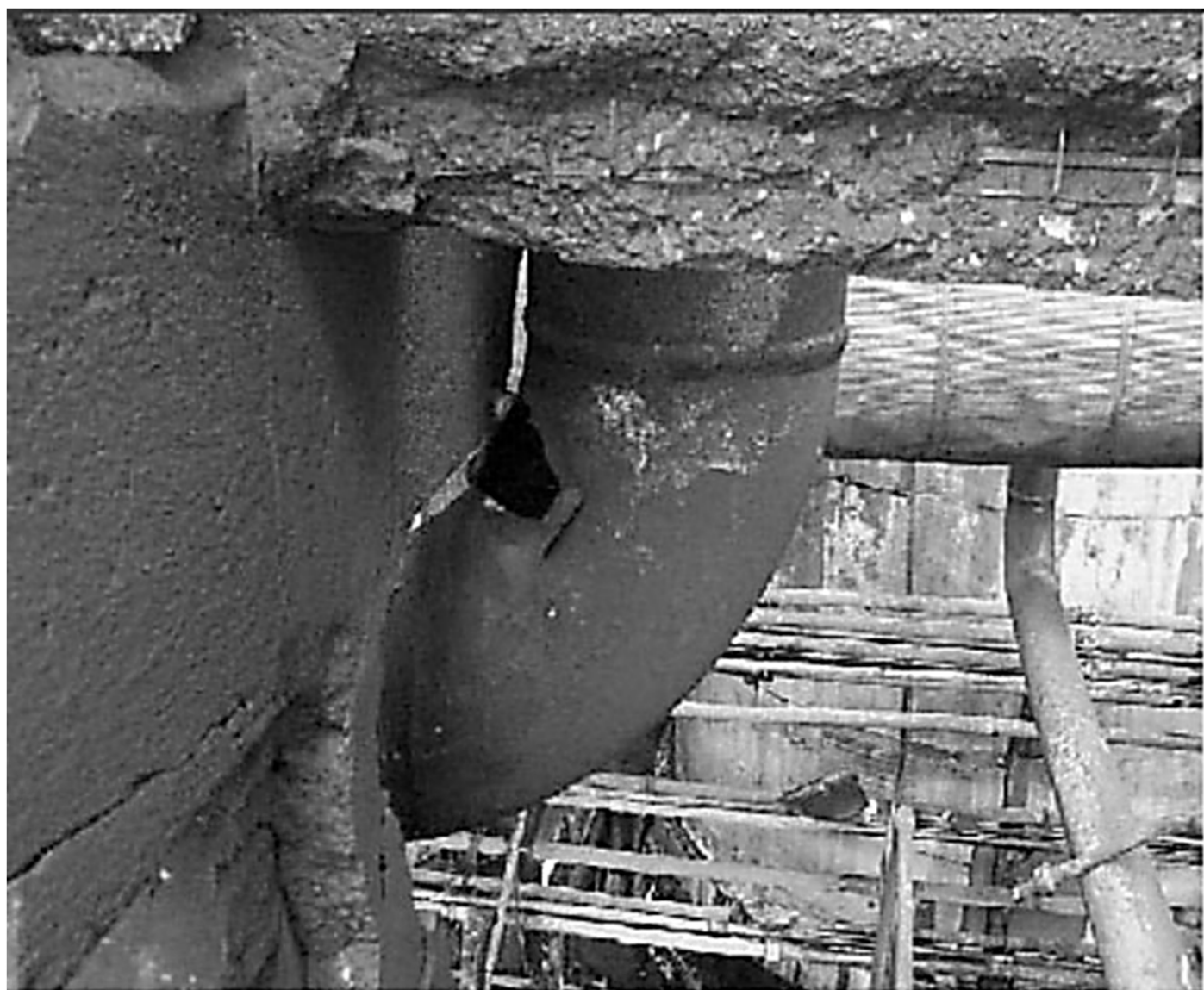
Figure 4-120 – Sulfidation failure of piping elbow.
