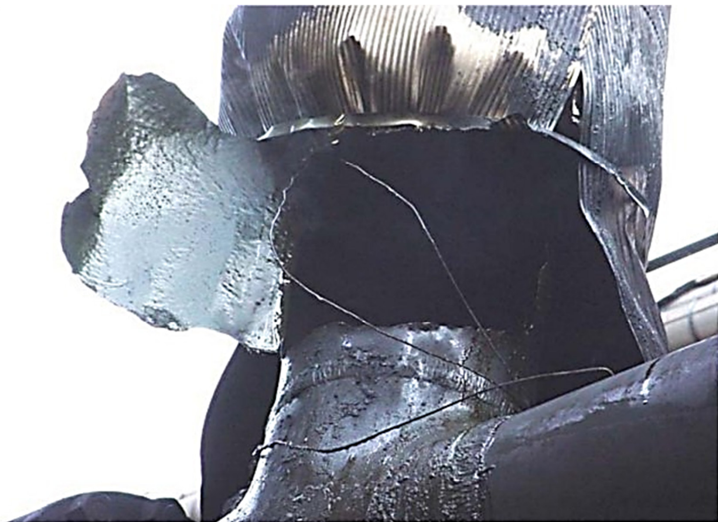
Figure 4-117 – Sulfidation failure illustrating the effect of accelerated corrosion due to low silicon content. This 8 inch NPS pipe section in FCC bottoms piping was in service at 150 psig (1Mpa) at 650° to 700°F (340° to 370°C). The piping sketch in Figure 118 illustrates the difference in corrosion rate as compared to adjacent high-silicon components.
