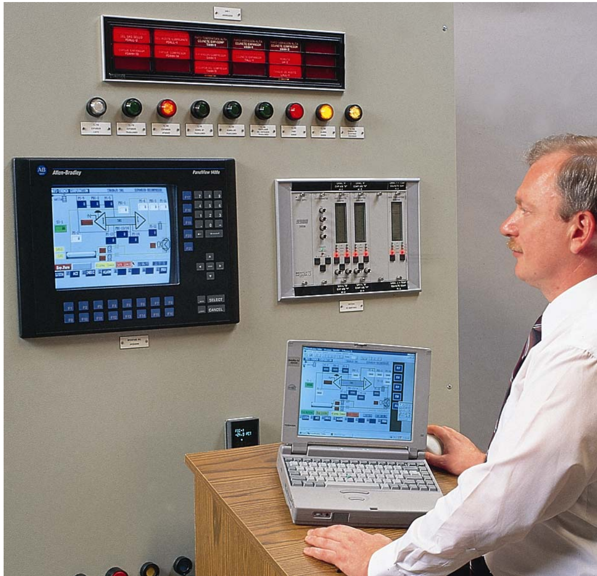
Remote PLC panel with Video Display Unit
