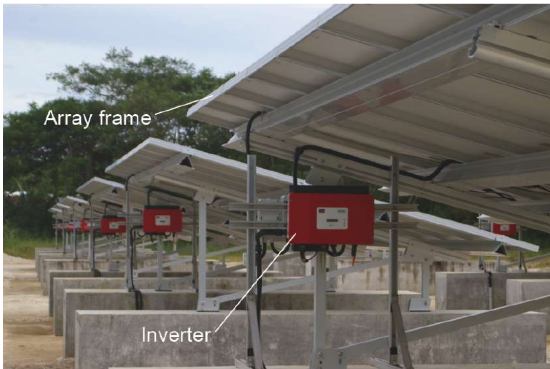
Figure 4: Showing Inverter and Frame
