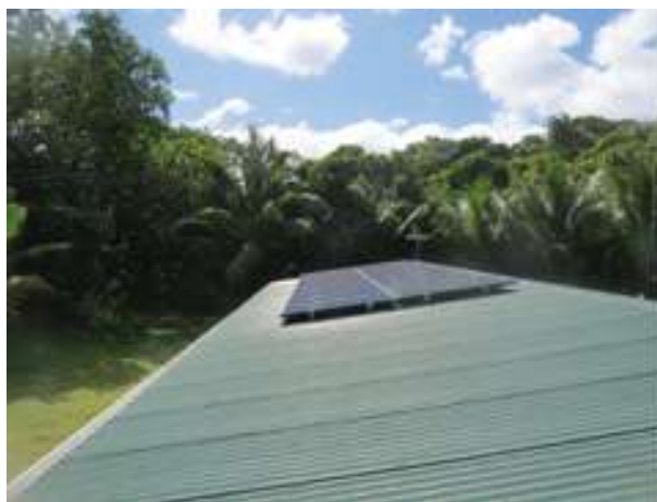
Figure 6: Array on House Roof
