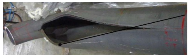
Figure 3: Photo of ruptured mixed feed piping
