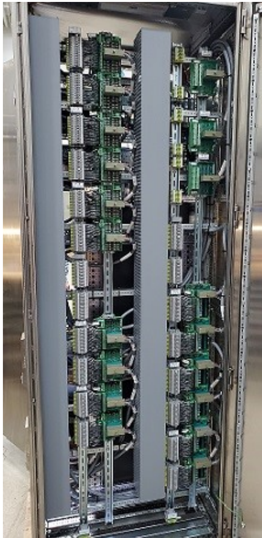
Figure 2: Back (I/O wiring) side of ESD control cabinet
