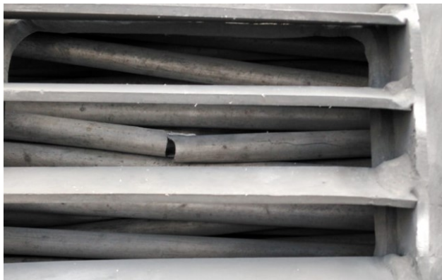
Figure 1. Broken tubes inside operated internal exchanger
