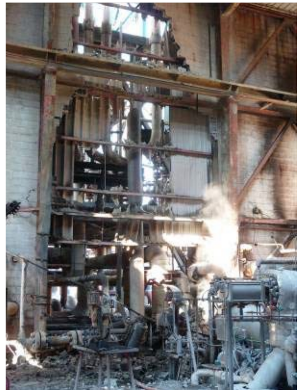
Figure 5. Compressor house after a fire
