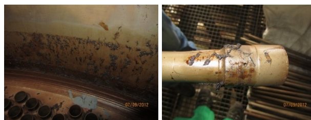
Figure 6: severe oil fouling top tube-sheet, blocking liquid inlet holes
