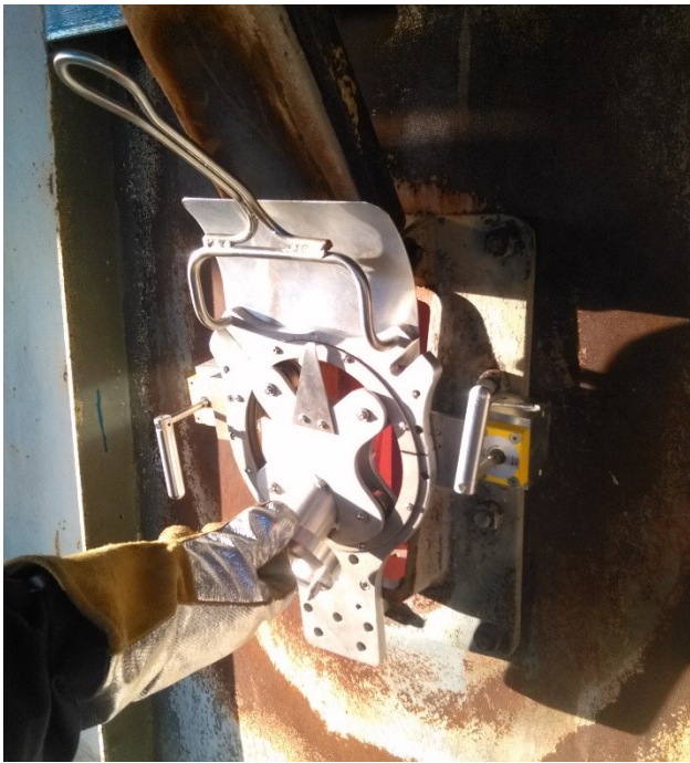
Figure 9. Photo of Reformer Imager Clamp in use on reformer peephole at Yara Le Havre.
