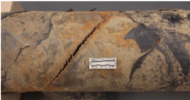
Figure 2. Corrosion Fatigue Cracking Rupture
