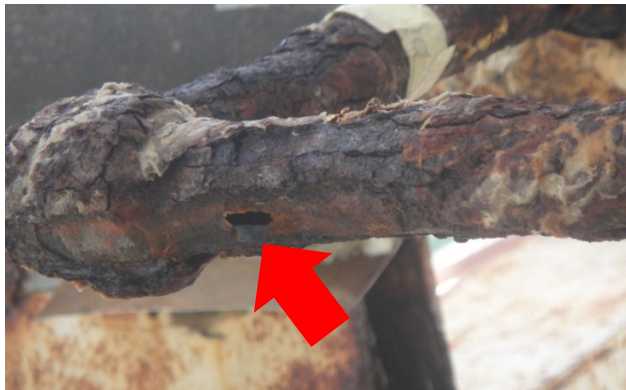
Figure 4. CUI on bypass MSV-0204
