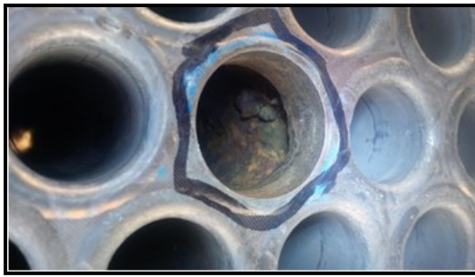
Figure 13. CP-Ti clad carbon steel tubesheet channel face and a location where a commercially pure titanium tube was removed.
