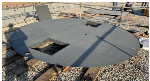
Figure 6. Temporary converter cover
