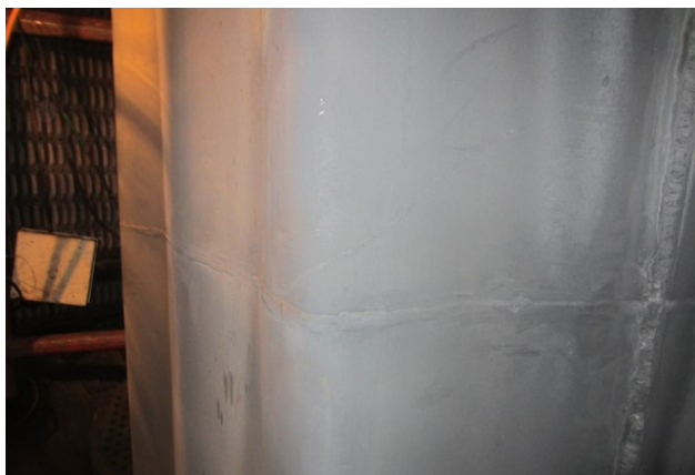
Figure 2. Deformed course inside an ammonia converter
