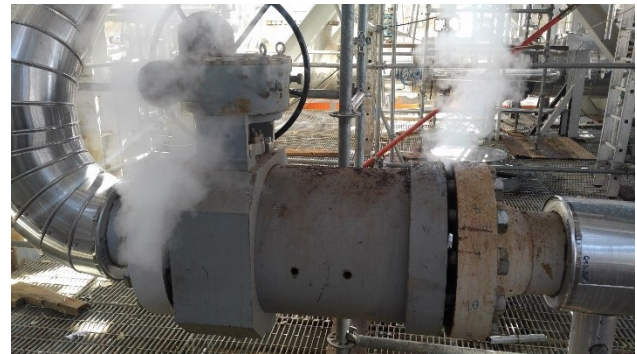
Figure 10. High-pressure steam valve leaking
