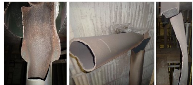
Figure 5: Photo of risers that were ruptured and dislocated
