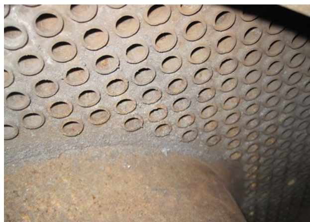
Figure 8. Oxidized surface of an operated internal exchanger
