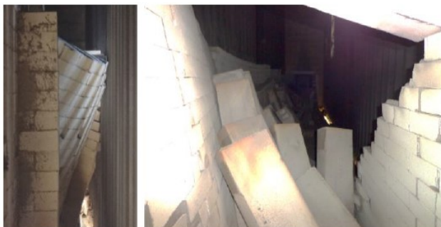
Figure 7: Photo showing significant damage to tunnel B walls and covers
