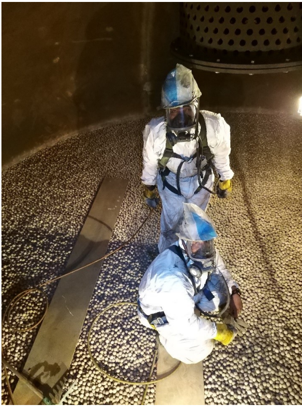
Figure 3. Loading crew with protective gear during final stage of HTS catalysts loading.
