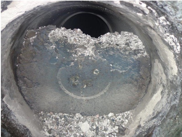
Figure 6: Photo showing refractory material and solidified molten metal deposited at the flanged end of the transfer line
