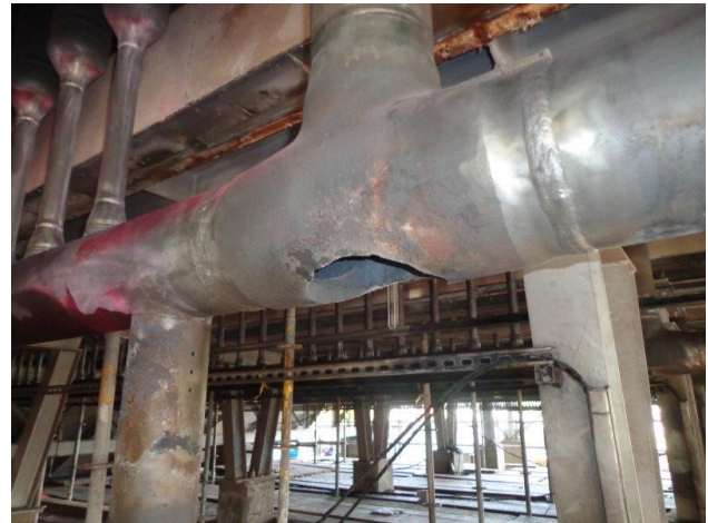
Figure 4: Photo of outlet header tee showing burn through due to reverse flow
