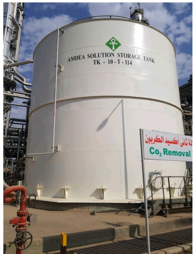
Figure 4. aMDEA Solution Storage Tank
