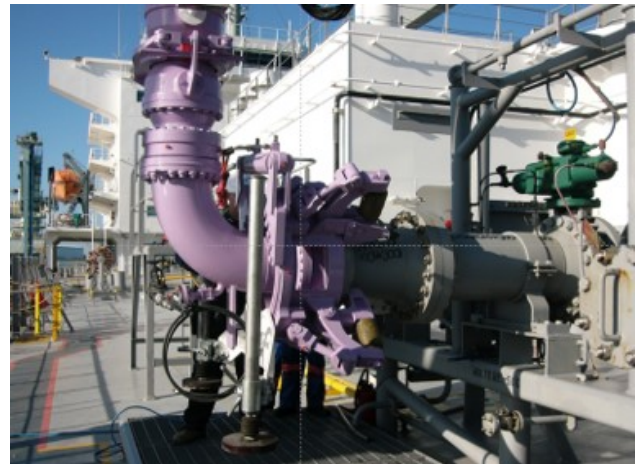
Figure 6. QCDC connection to ship manifold
