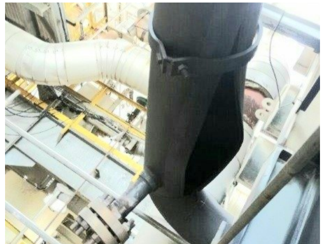
Figure 2: Photo of ruptured mixed feed piping
