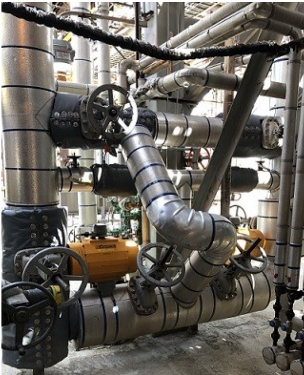
Figure 6: Reformer fuel isolation valves with online testing bypass
