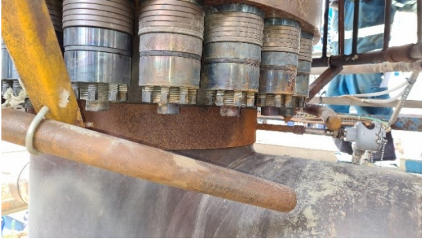
Figure 2. Modification implemented in Bottom Flange of the Synthesis Reactor – Superbolts® and spring washers.
