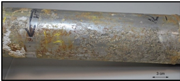
Figure 10. External Pitting due to CUI on Type 304/304L stainless steel NPS 3 pipe
