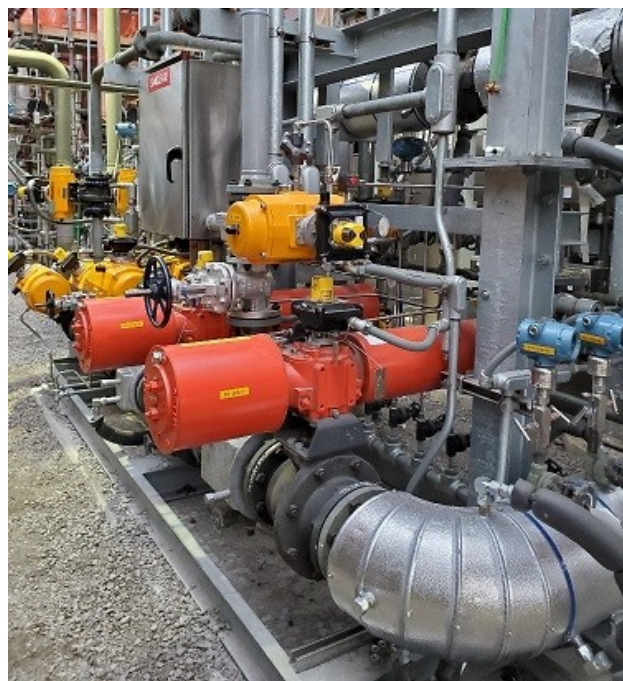
Figure 5: Input and output devices on a skid
