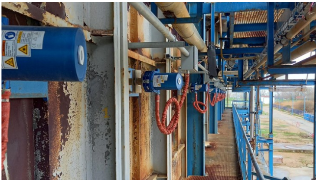
Figure 10. Photo of installed ZoloSCAN sensor heads on the reformer at Yara Le Havre.
