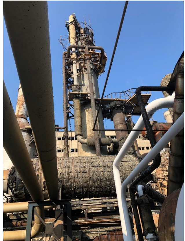
Figure 6. Synthesis loop fire aftermath due to pipe rupture.
