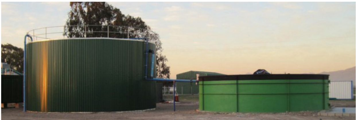
Figure 2.8: Zandam Farm plant (Anaergia)
