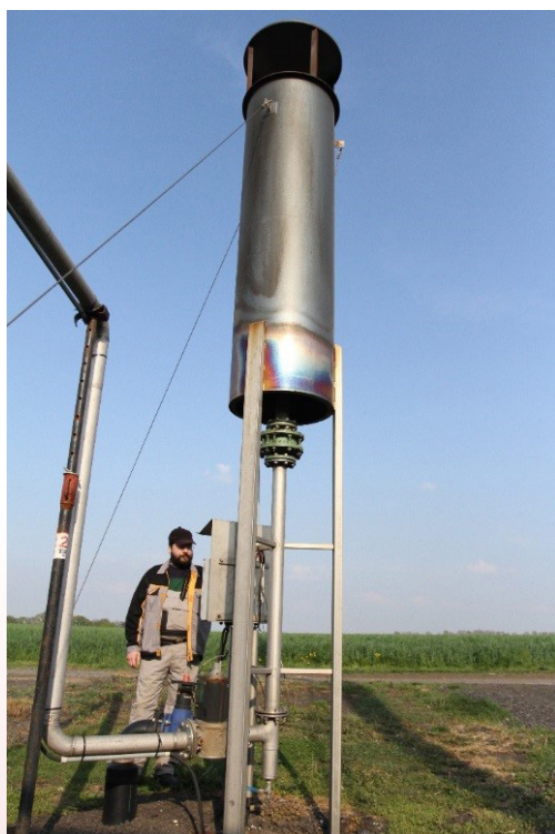
Figure 6.11: Gas flare of a biogas plant (Anaergia)
