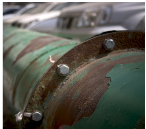
Figure 91: Poor adherence of the paint
