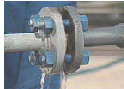
Figure 70: Leak on a water pipe flange
