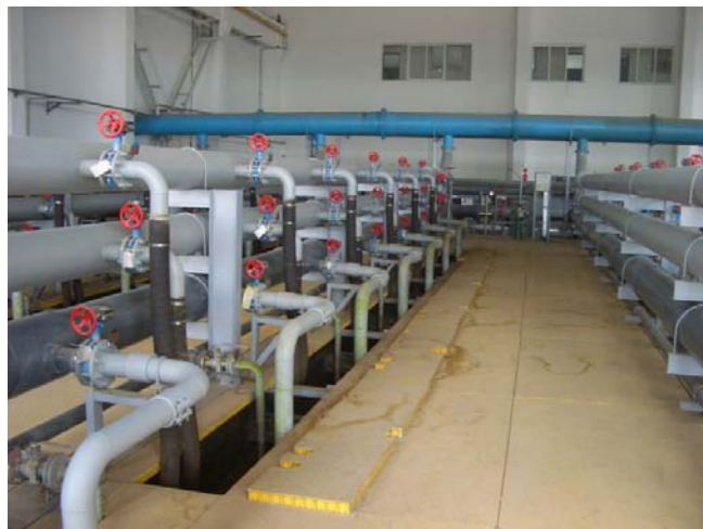
Figure 14. The membrane tank in Golden Bridge power plant, Hohhot.
