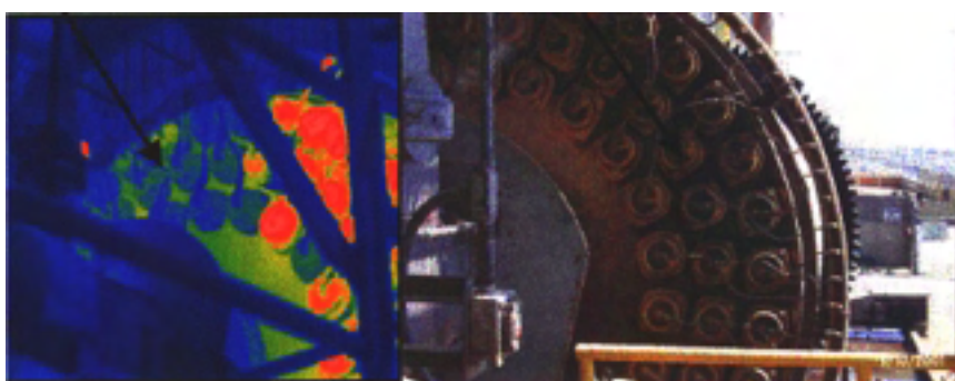
Figure 6.2.9. Inoperable steam heaters seen by cooler blue areas when compared to the operating heaters warmer red or orange colors.
