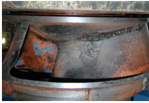
Figure 13: On this impeller, cavitation damage is located near the hub on the pressure side of the blade. In this case the pump has been operated in the recirculation region; matters have been worsened with speed variation and a flat system curve.
