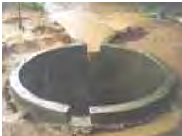
Figure 18. Run off rain water collection to the tank.
