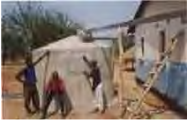
(a) Rainwater harvesting from roofs provides clean drinking water for domestic use and small livestock.
