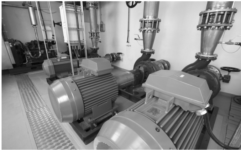
Figure 13. Pressure boosting station in Pietarsaari, Finland.
