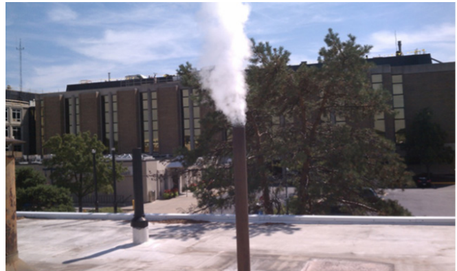
Figure 10. Example of steam plume from a roof vent, indicating a failed steam trap.
