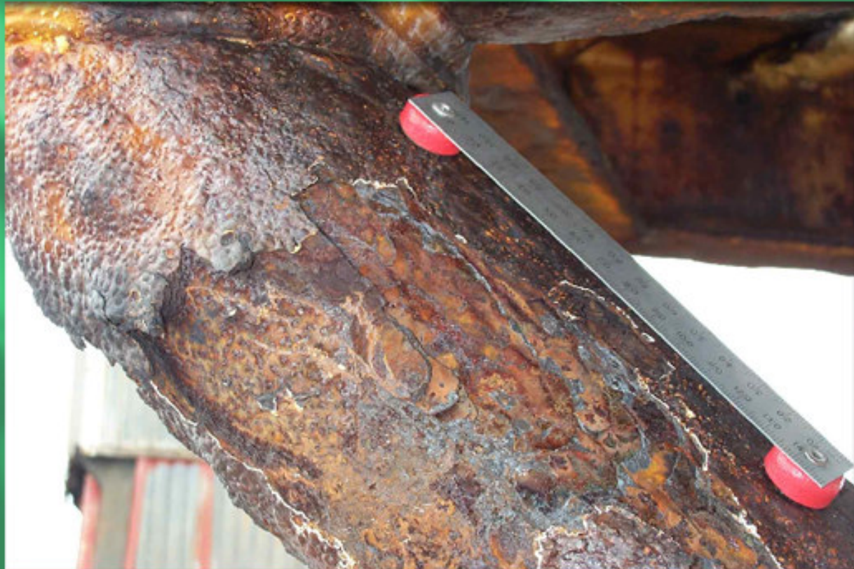
External corrosion of structural steel work
