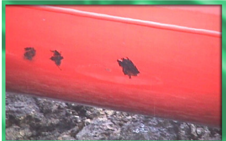
Damage to New Coating
