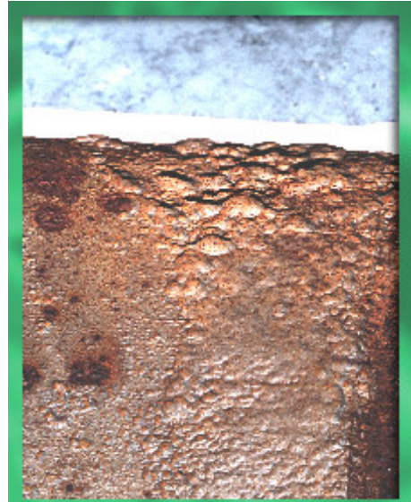
\text{CO}_2 corrosion of carbon steel
