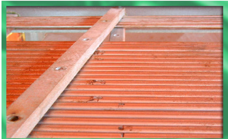
Corrosion of Stainless Steel Impulse Lines
