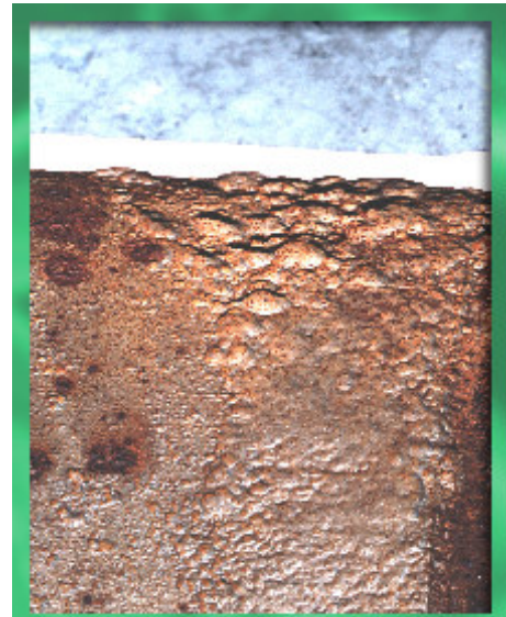
\text{CO}_2 corrosion of carbon steel
