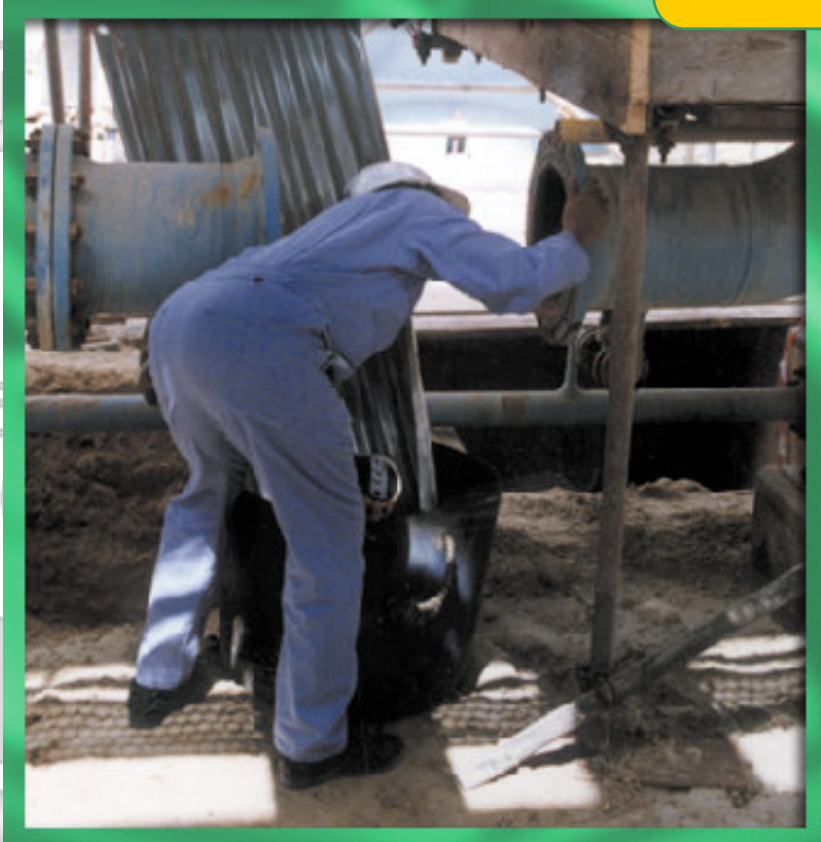
Maintenance work - When opening up pipework, look inside and report concerns
