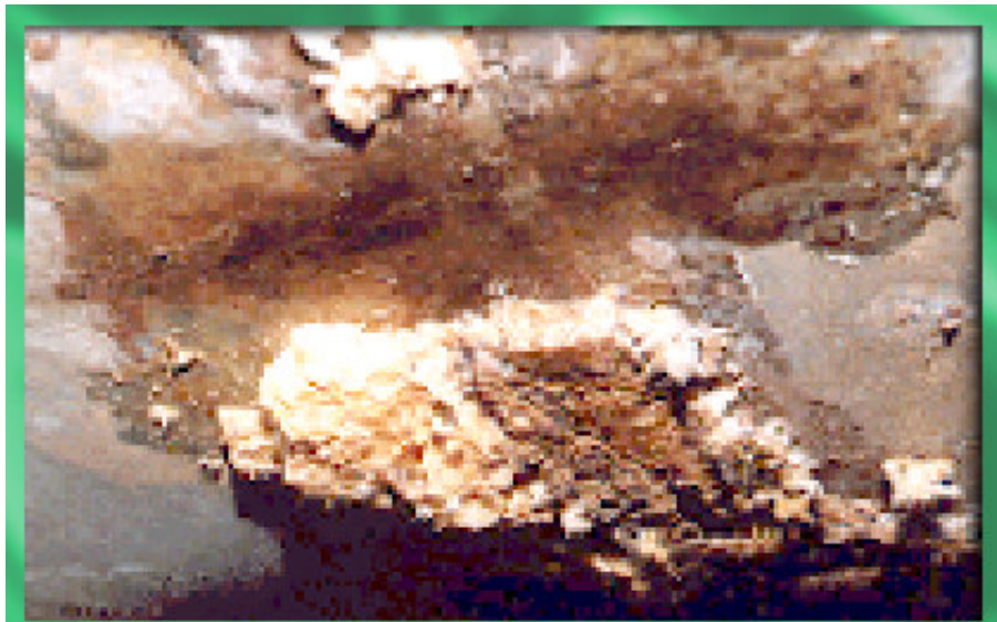
Corrosion of Stainless Steel Separator
