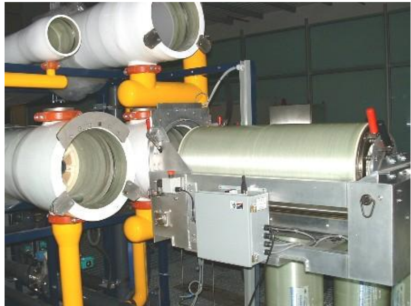
Loading tool attached to 16-inch pressure vessel
