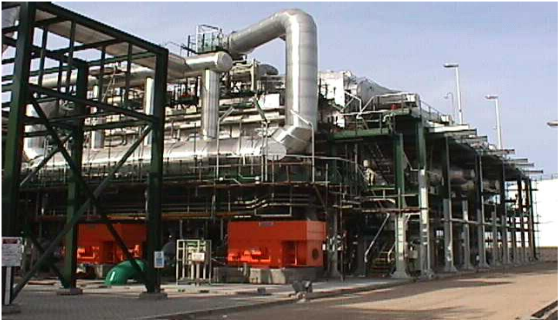
MSF 5 MIGD Layyah Plant subject of Integrated Upgrading
