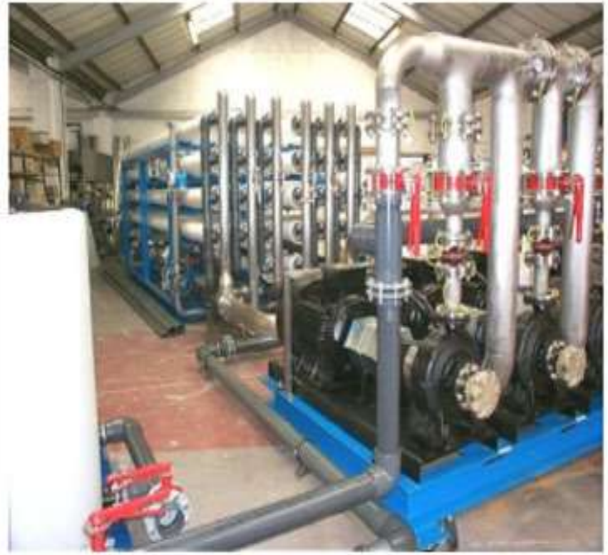
4200 m 3 /day Reverse Osmosis Unit for Industrial Water Application
