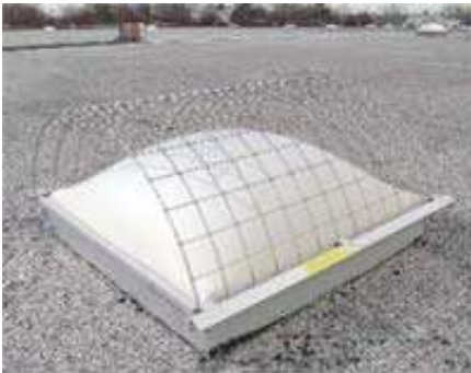
This photo shows a skylight guard
