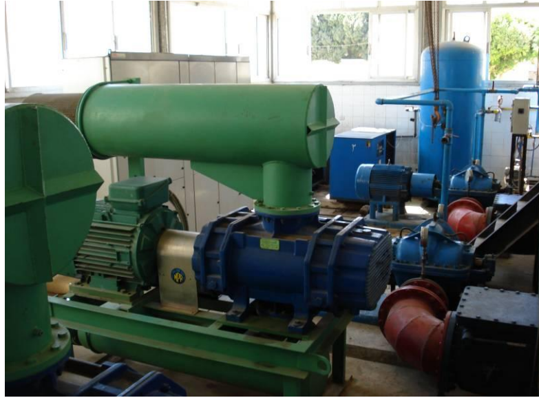
Picture 4 – Qus WTP: O&M manuals should be available for this type of equipment.
