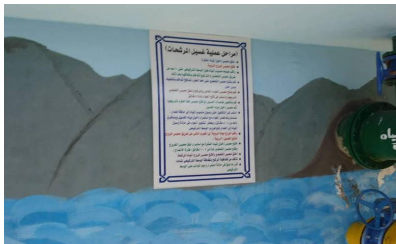
Picture 3 - Filter Washing Procedure at El Toyrate New WTP
