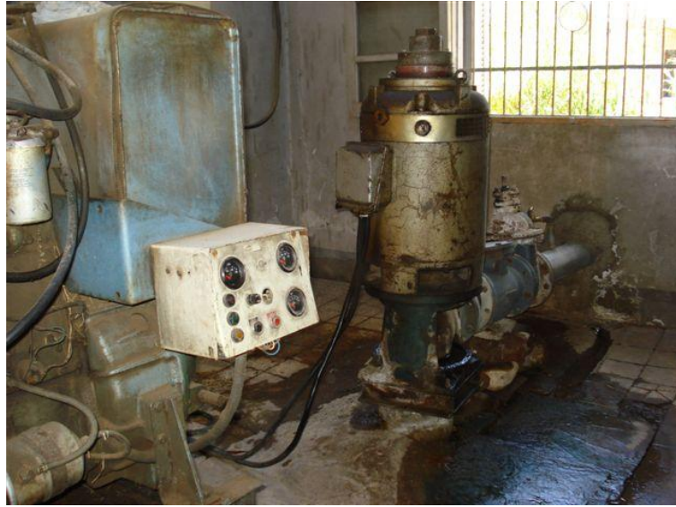
Picture 1 - A Typical Ground Water Source at Gezeret Dandra
