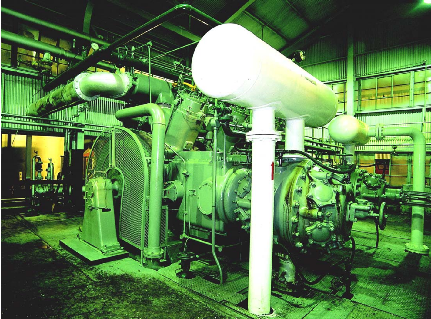
Combined gas engine / compressor with manual clearance pocket capacity control (USA)
