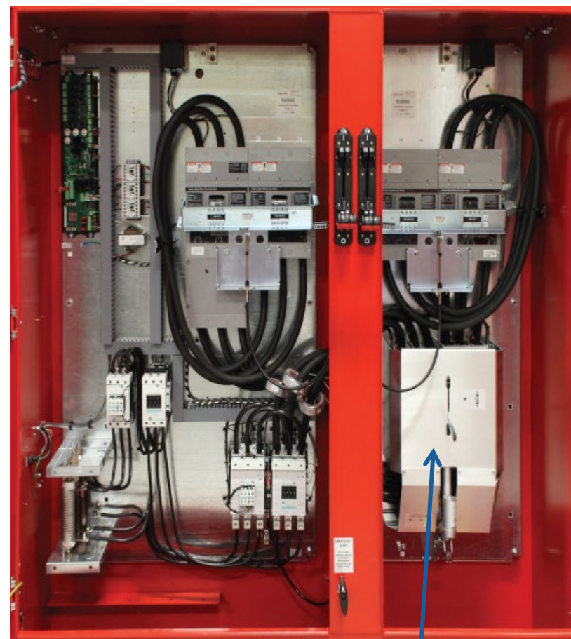
Automatic Transfer Switch
