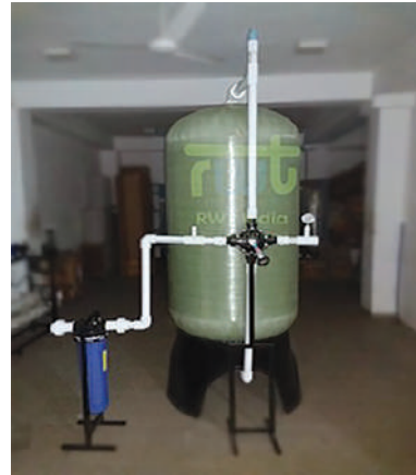
Figure 9: Pressure sand filter (PSF)
