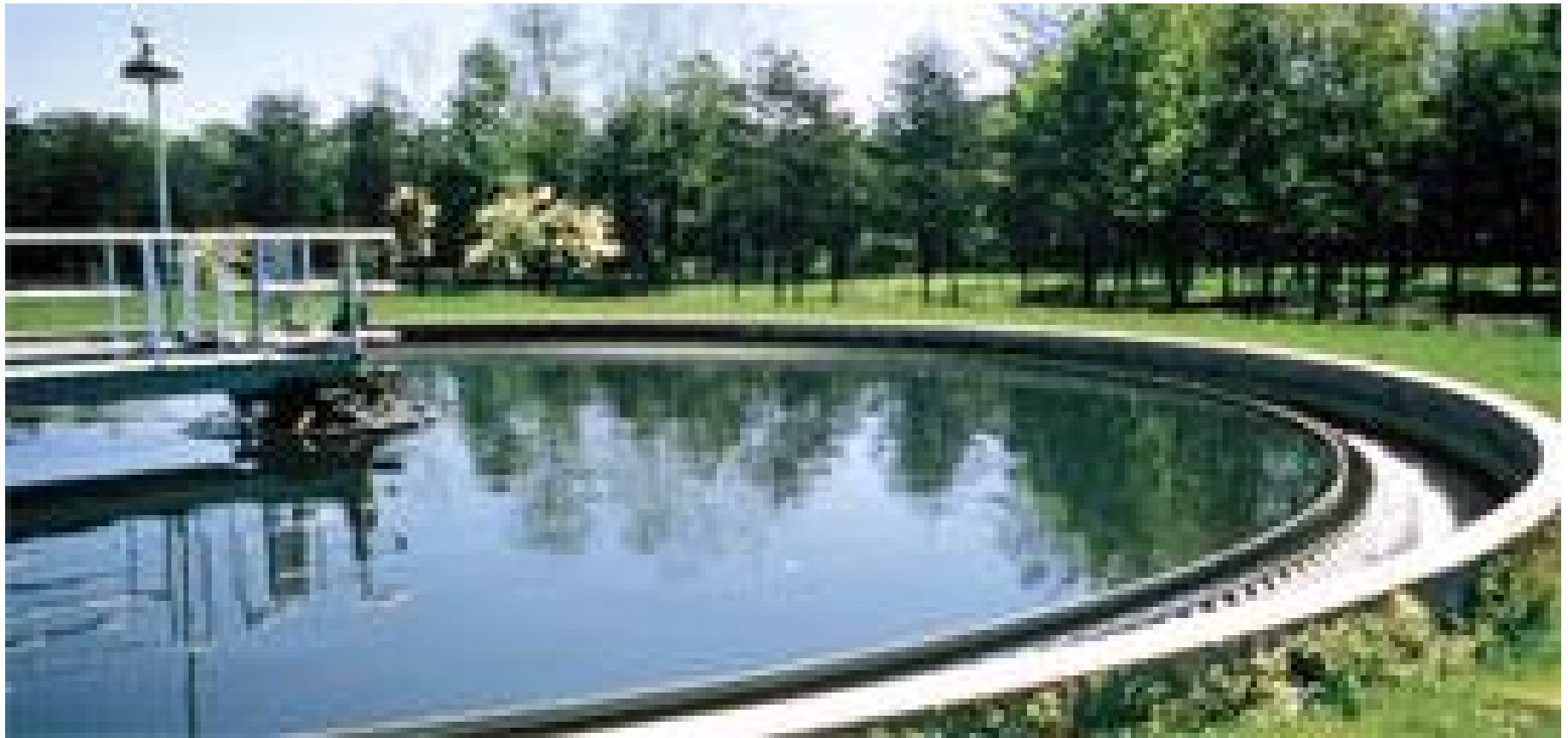
Effluent channel of circular sedimentation basins.
