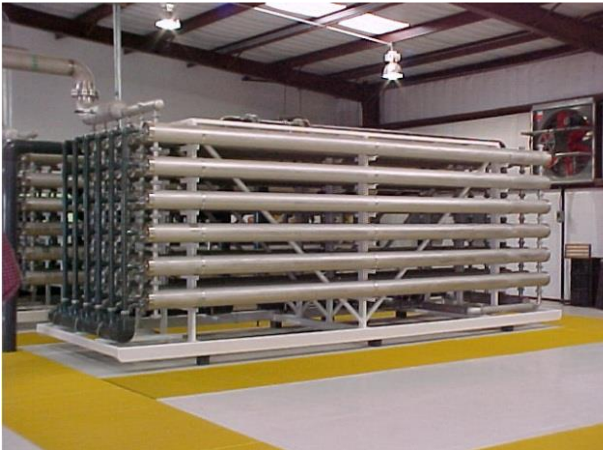
Fig 4.2 Reverse Osmosis plant
