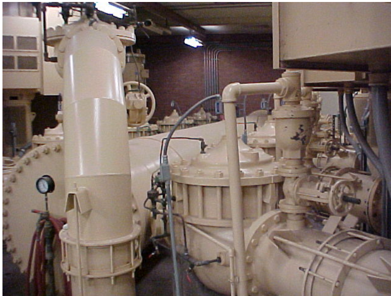
The inside of a booster pump station, notice the PRV with air relief valve.
