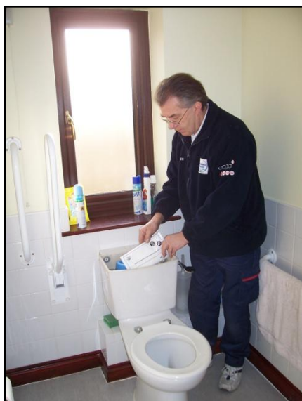
Plumber fits a save-a-flush bag to a toilet cistern (image courtesy of Thames Water)
