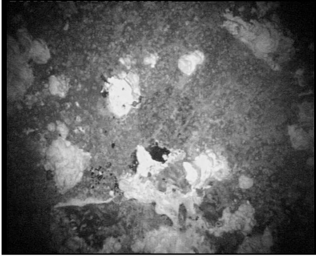
Figure 3 Photo of the internal surface of a corroded iron pipe showing scattered corrosion nodules
