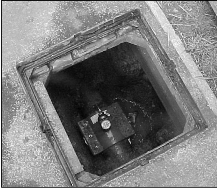
Figure 2 A typical chamber with a 2-in. gate valve installed for the inspection using the trunk mains sampler
