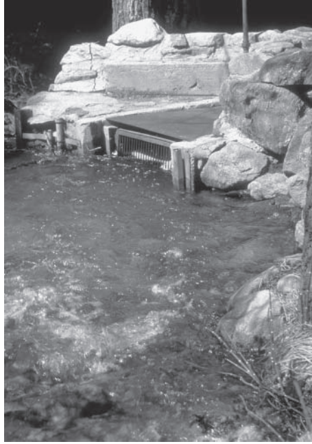
Drinking water intake, E. Fork Santa Ana River, California
