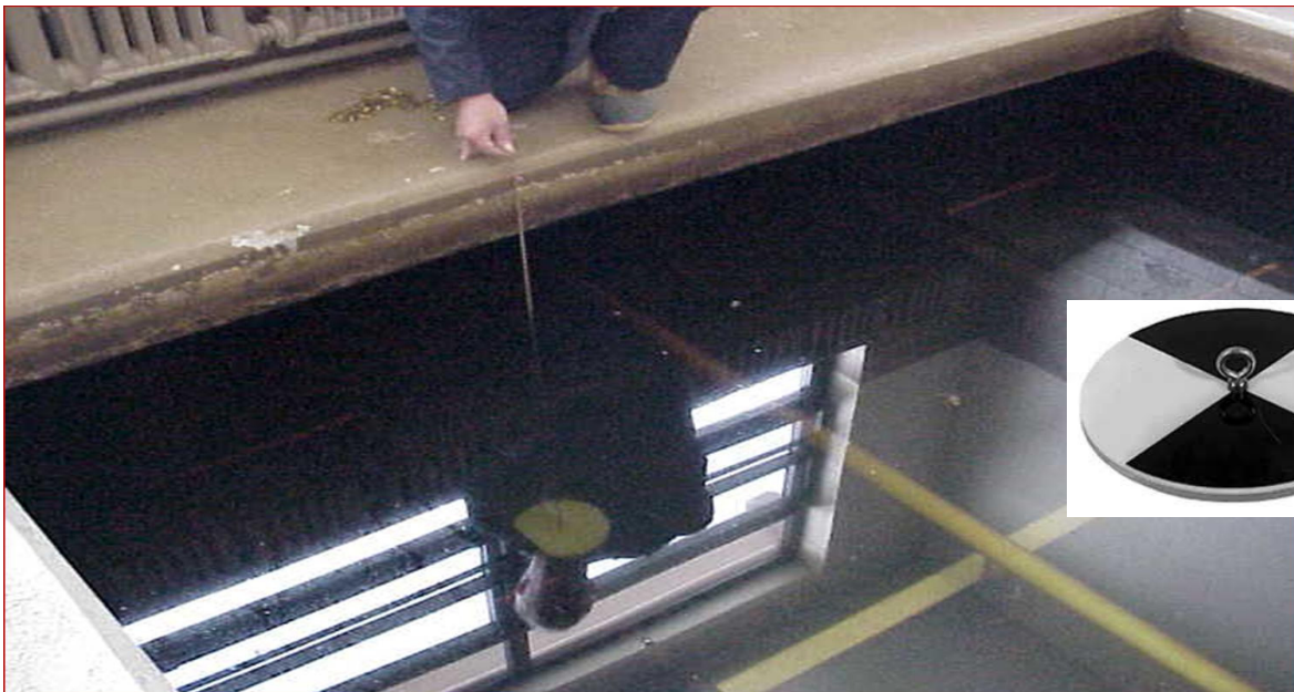
Determining Filter Bed Expansion with a SECCHI DISC
