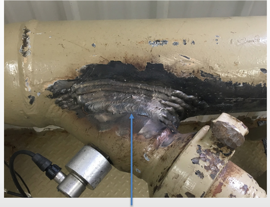
Location of Previous Failure
