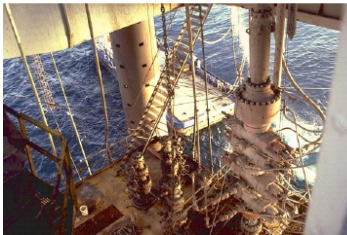
Figure 61 BOP on Cellar deck
