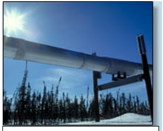
Figure 116 The 48" diameter Alyaska Pipeline delivers 1 million barrels per day of crude oil. That would fill a Very Large Crude Carrier (VLCC) in 2 days.
