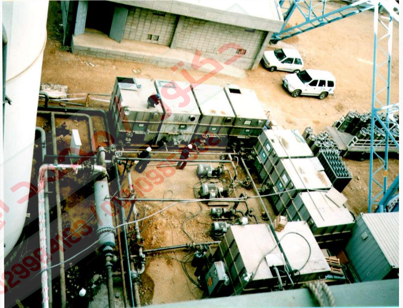
Chemical washing equipment area
