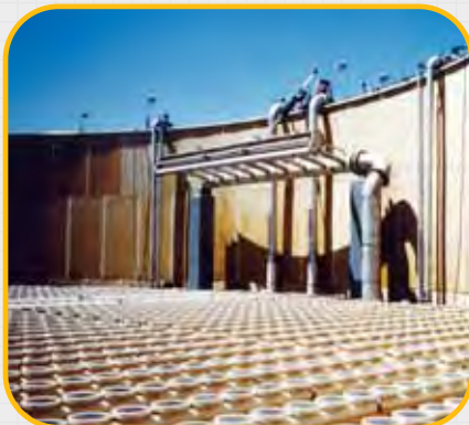
Industrial wastewater treatment plant in circular tanks
