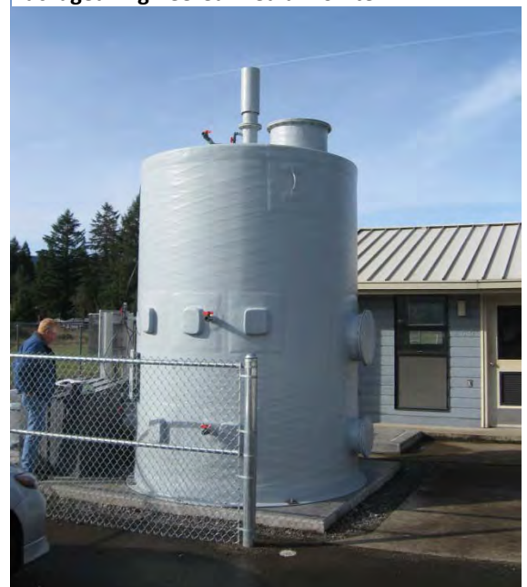
FIGURE 16-5 Packaged Engineered Media Biofilter
