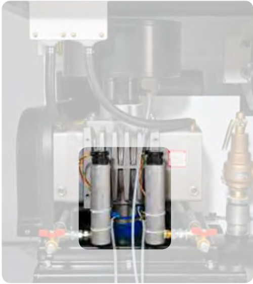
Oil level sensors and oil temp sensors
