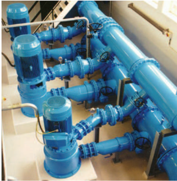
Figure 15 - Pumps used for the transportation of drinking water
