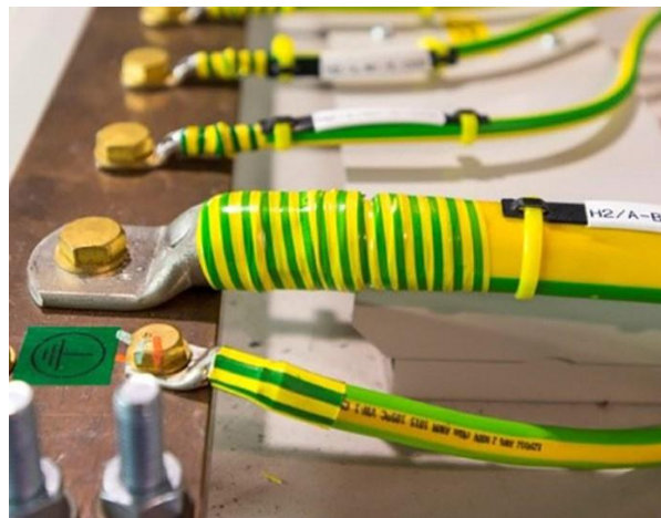
Figure 7: Marking of Earth Conductors
