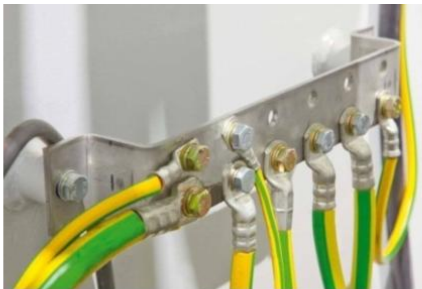
Figure 21: Main Earthing Terminal (MET)
