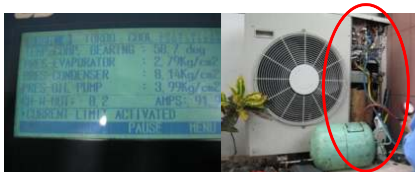
Figure 57. HVAC system data collection
