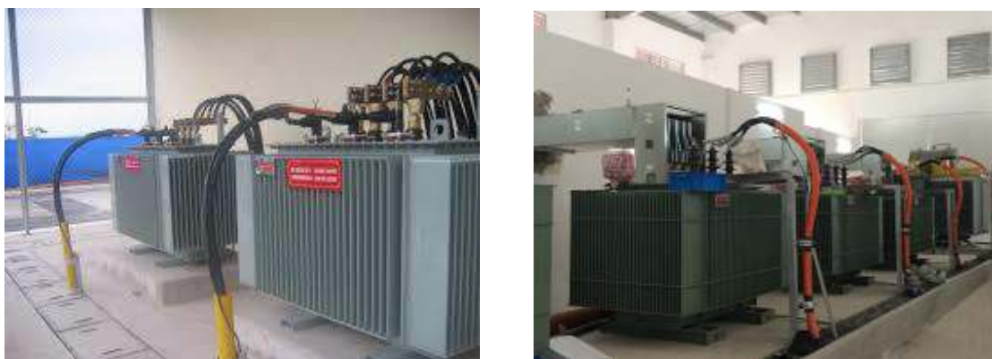
Figure 10. The transformer in power system
