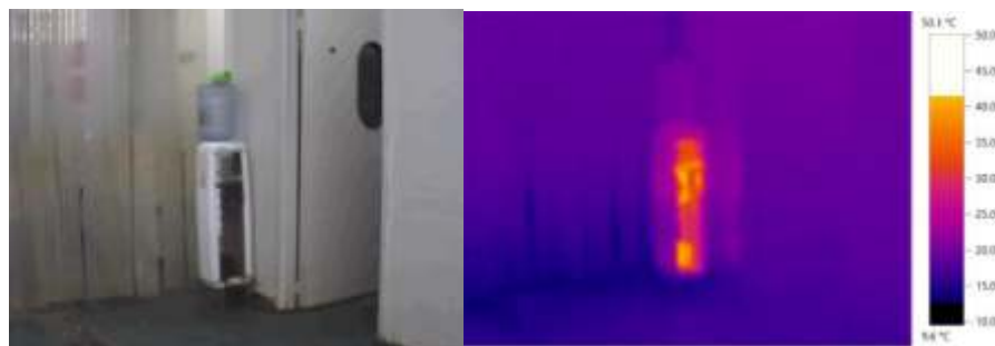
Figure 59. Detect heat sources inside HVAC space
