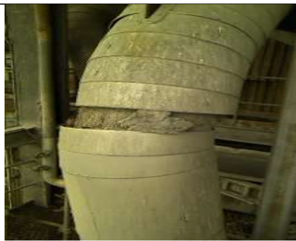
HRH near boiler drum floor
