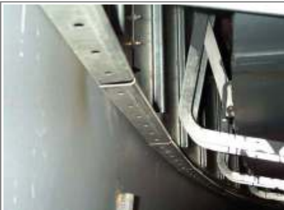
The end section of WB-1 mechanical shoe seal and counter weight
