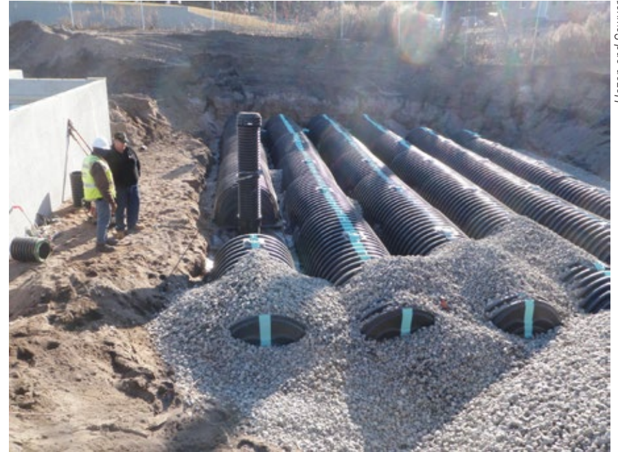
Perforated pipes in New York, NY.
