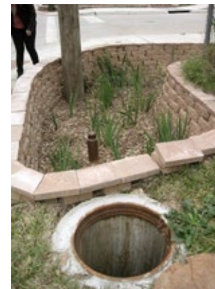
Figure 4-27. To facilitate maintenance, an observation well is installed next to a bioretention area in Houston, TX.
