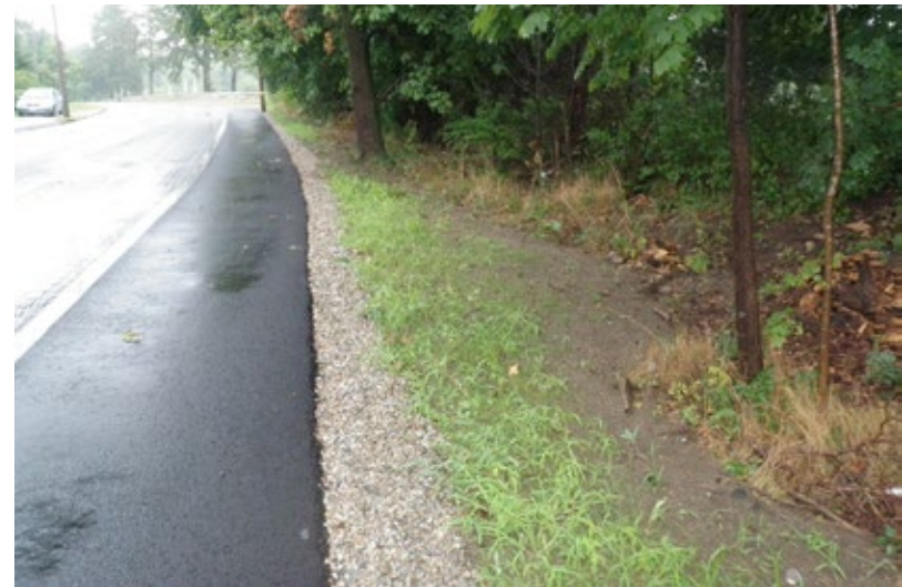
Infiltration trench (gravel) adjacent to a roadway.
