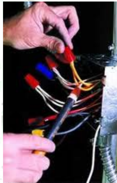
Always test a circuit to make sure it is de-energized before working on it
