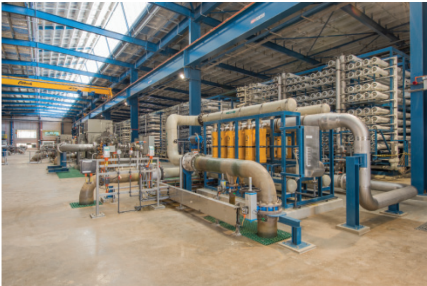
Figure 10. ERI pressure exchange energy recovery units.
