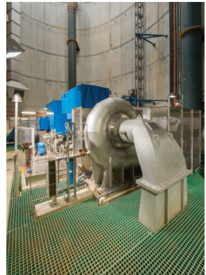
Figure 11. Energy recovery turbines.
