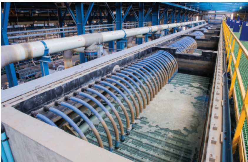
Figure 9. The ultra-filtration plant.
