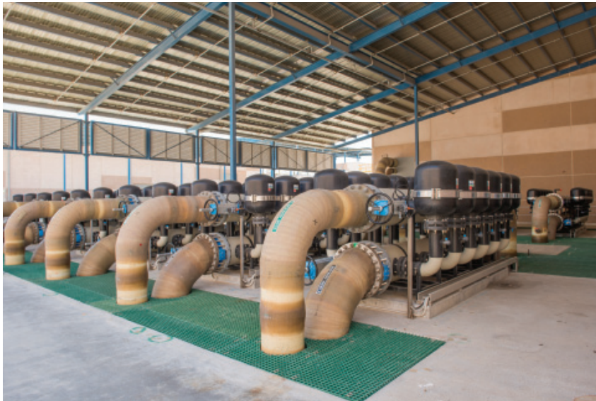
Figure 8. Disc filters at the main process plant.
