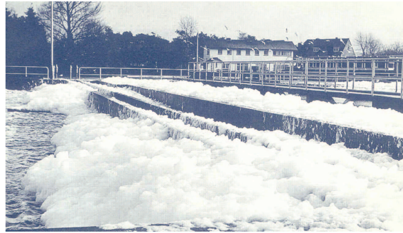
Figure 4 - In the seventies, water contained detergents resulting in foaming in wastewater treatment installations
