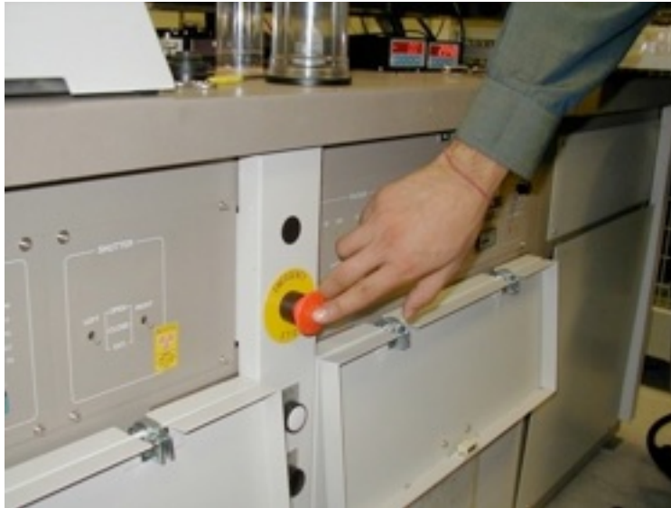
Fig. 5.3.1.b – An Emergency Stop (E-Stop) does not cut all electrical power to equipment.
