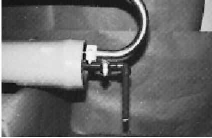
Picture 1: Disconnecting Ports
