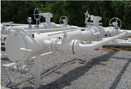
Fig 32. Inline Inspection Pig Launcher
