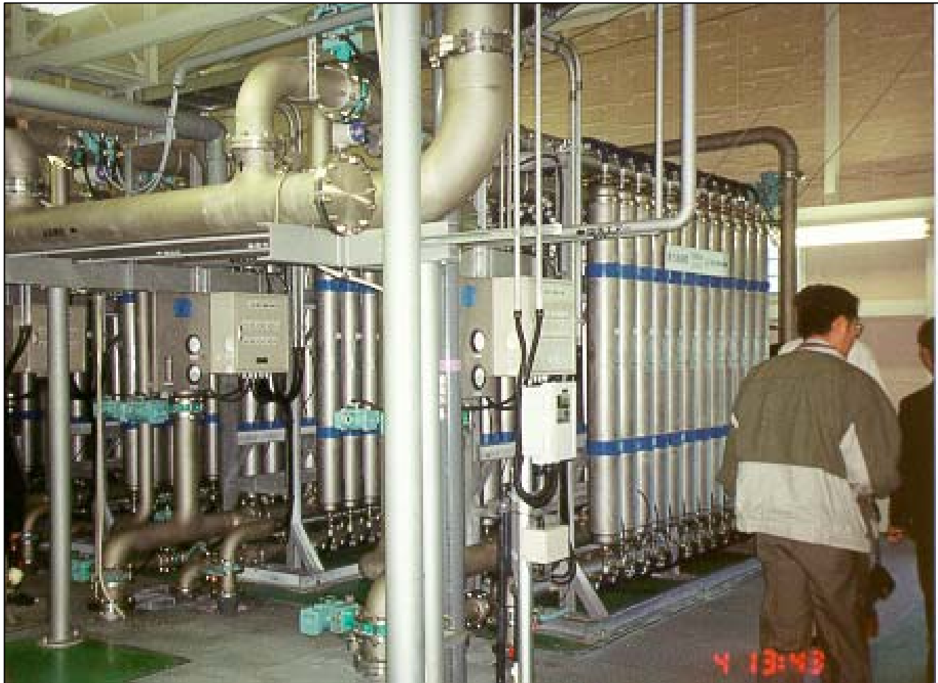
Membrane plant for water treatment, Ogose Town, Japan
