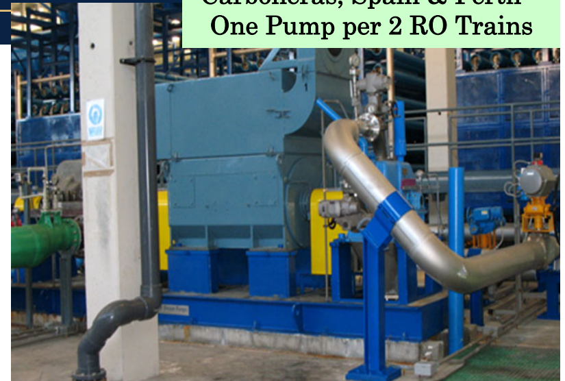
Ashkelon, Israel – Two Pumps per 16 RO Trains
