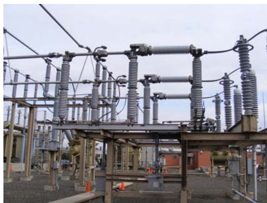
Fig.11. 230 kV 1200 A Circuit Switcher Substation Bus Systems
