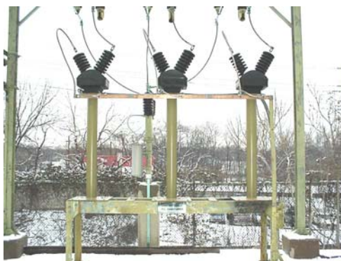
Fig. 21. 26 kV Potential Transformers
