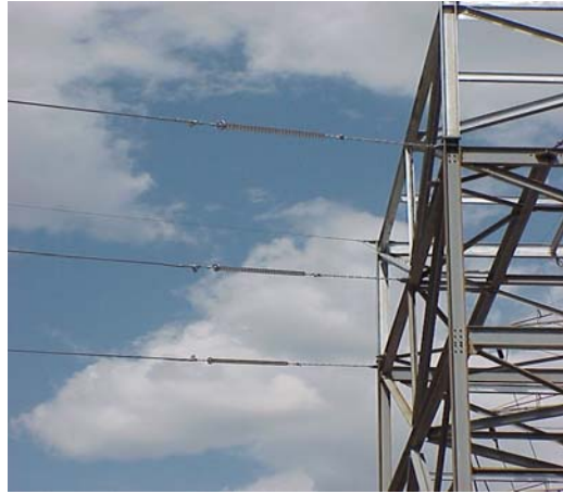
Fig. 15. 230 kV Strain Insulator Assembly
