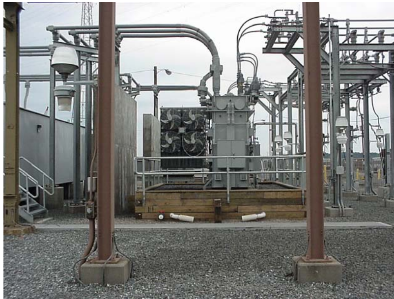
Fig. 3. 13/4 kV 6.0/9.0 MVA OA/FA Transformer
