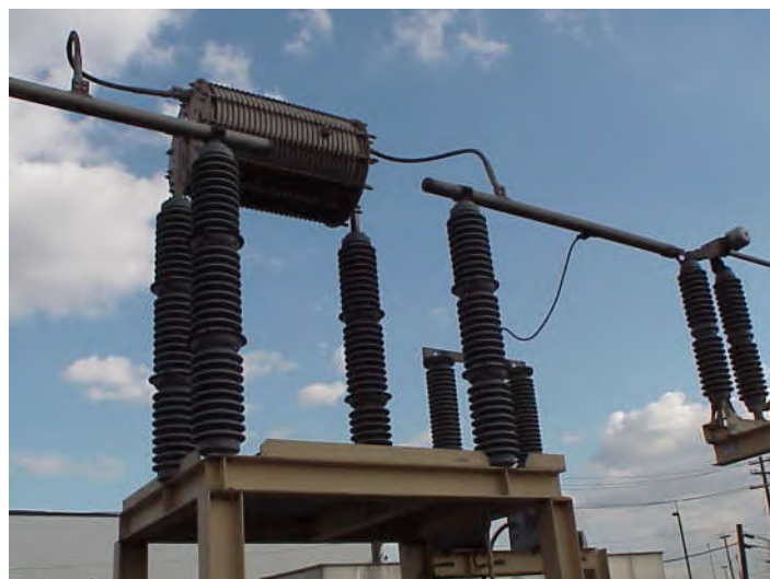
Fig. 13. Free Standing 138 kV 2000 A Wave Trap
