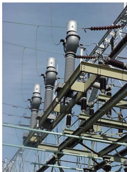
Fig. 18. Free Standing 138 kV 2000/5 A CTs
