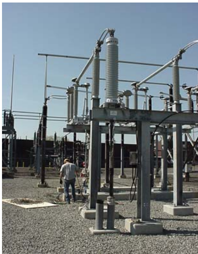
Fig. 17. 138 kV Solid Dielectric Cable Bus Terminal
