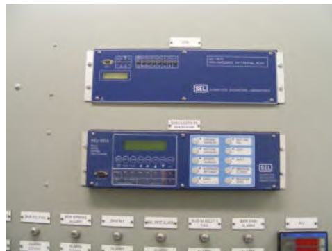
Fig. 2. Microprocessor Relays Installed on the Panel
