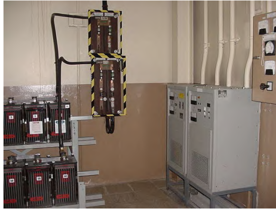
Fig. 18. Substation Auxiliary DC Equipment
