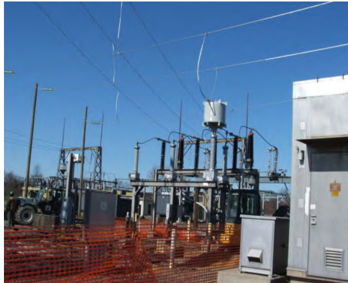
Fig. 12. 138 kV CCVT with 3000 A Wave Trap
