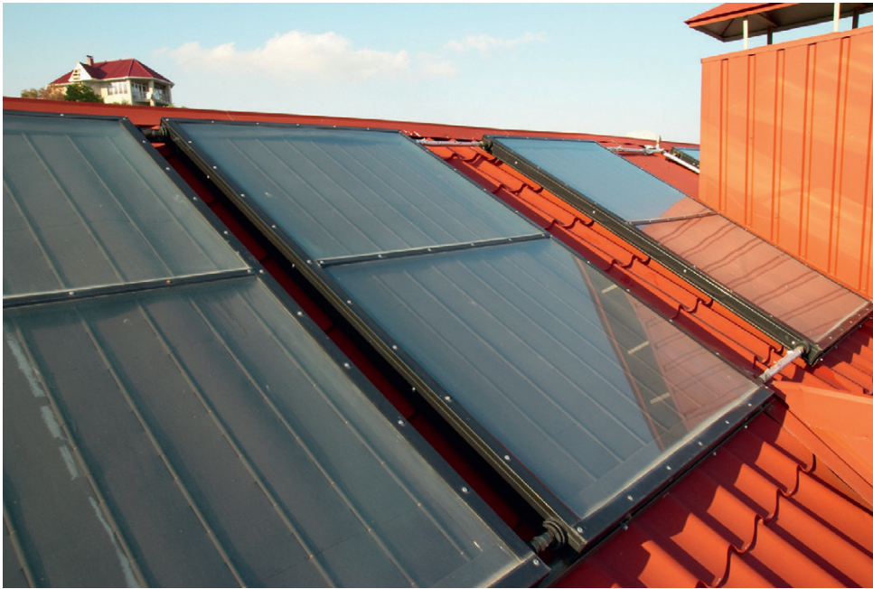
Figure 5.3 Photograph of a solar hot water panels.
